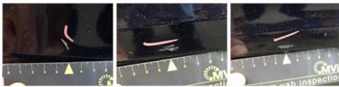
Door R R, Bad repair, Acceptable
